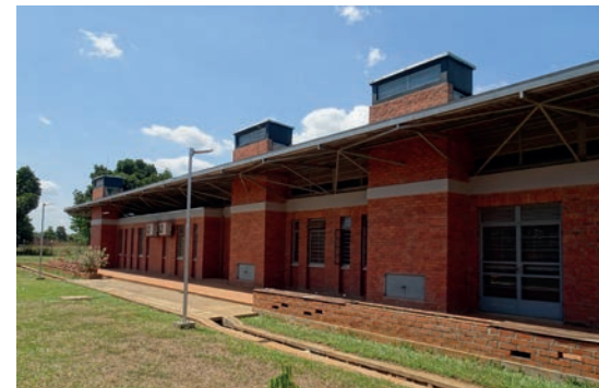
NTC Kaliro Solar chimneys were designed incorrectly and consequently failed to provide a significant stack ventilation effect
