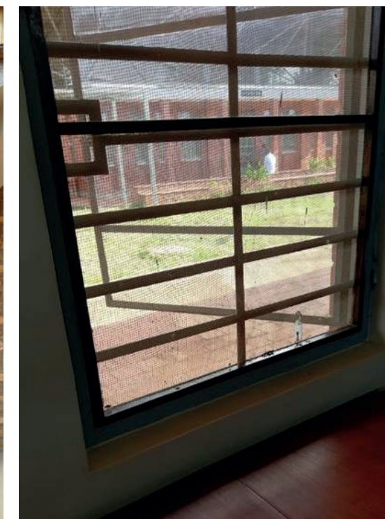
NTC Kaliro A layer of framed mosquito netting can be opened or closed independently of the glazed windows
