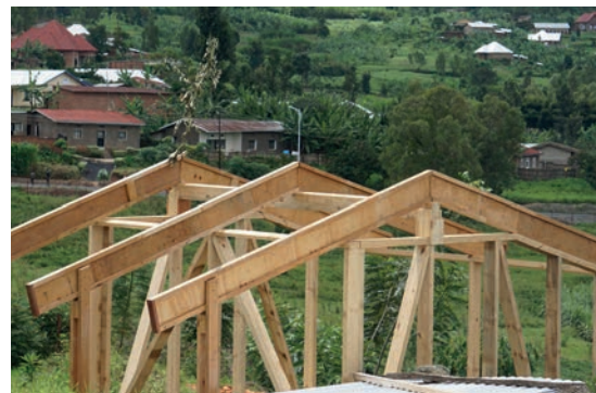
At the Rubengera Technical School, Rwanda, they are experimenting with laminated timber as well as I-section timber beams
