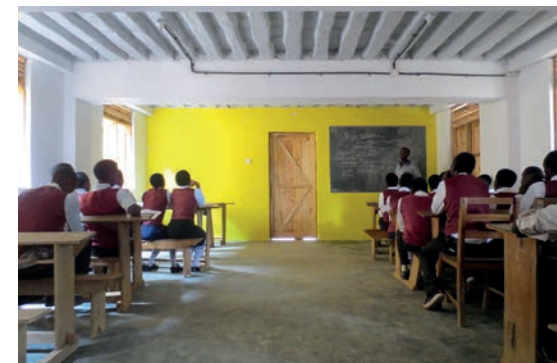
Lake Bunyonyi Secondary Bricks were inlaid into the first floor formwork to reduce the amount of concrete required
