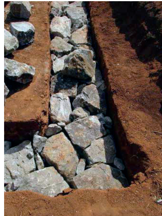
AWF Primaries The schools are built on traditional rubble stone foundations - without the use of concrete
