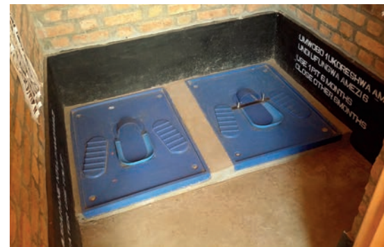
ECD&F Centres use ecological sanitation technology to improve hygiene and comfort by reducing smell and sealing from flies
