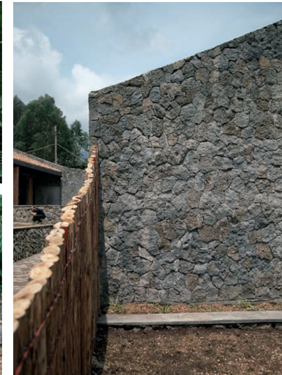
Ruhehe Primary Scaffold poles from construction were upcycled into play equipment, water tank screens and fences
