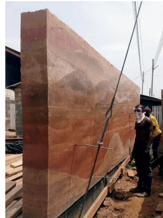
Fresh rammed earth wall produced by Hive Earth - a specialist earth construction company based in Ghana
