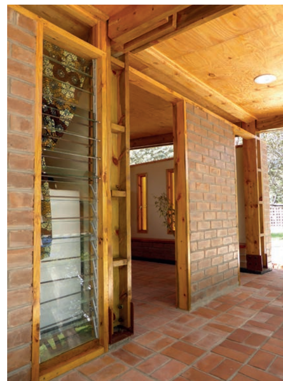
Mzuzu Health Centre Mechanical glazed louvres provide both natural daylighting and passive ventilation
