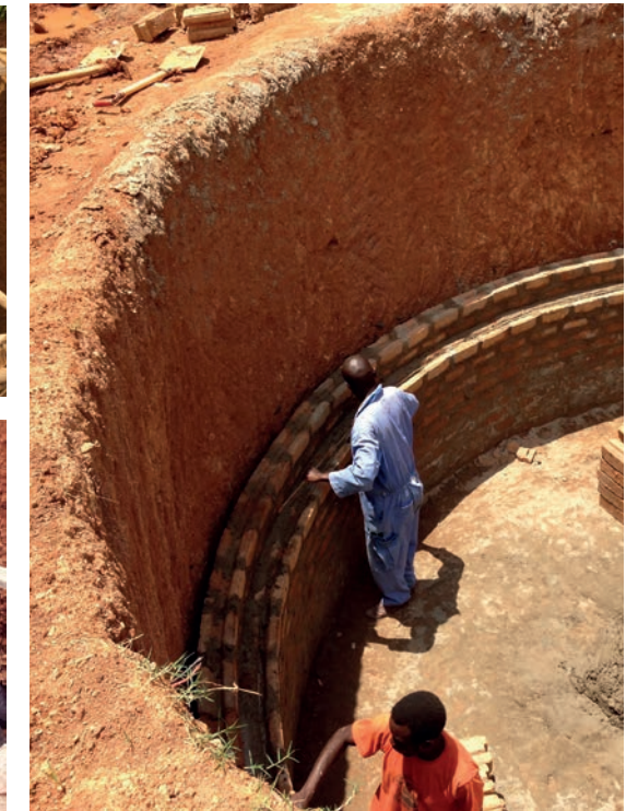
A large ISSB water tank consisting of two concentric circles of standard ISSB for additional reinforcement
