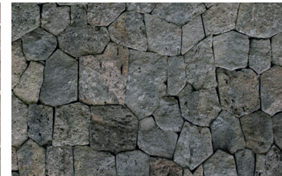
Ruhehe Primary Volcanic rock is built around a central core of steel and concrete to guarantee stability
