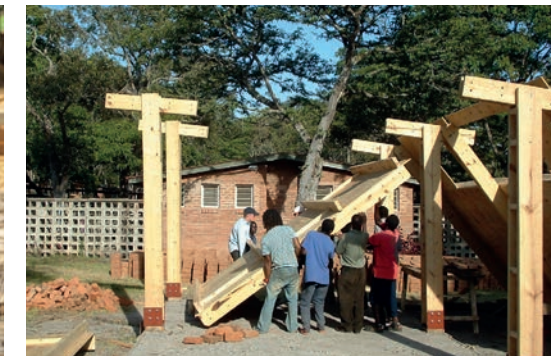
Mzuzu Health Centre The project focus was to provide the client with their own highly affordable DIY construction system
