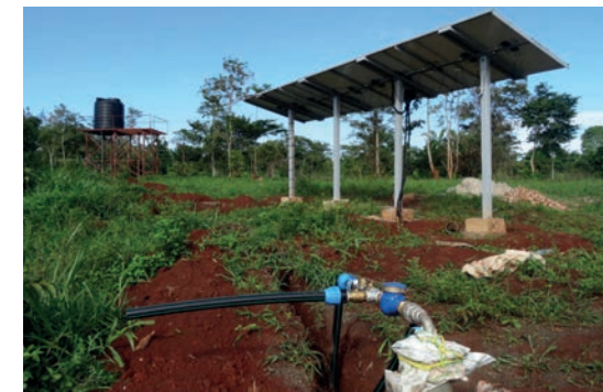
Good Future and Hope have installed a solar-powered borehole and 10,000L storage tank at their orphanage in Nakisunga, Uganda
