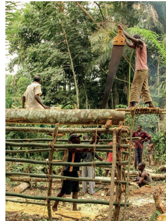
Ilima Primary has virtually no embodied energy - built entirely with simple hand tools and local materials
