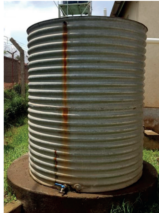
A corrugated iron water tank showing signs of rust
