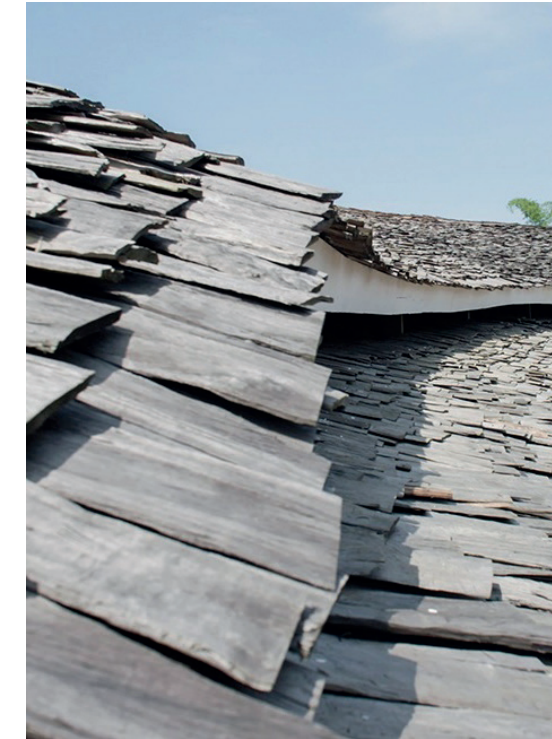
Ilima Primary Locally harvested timber was transformed by hand into durable and replaceable hardwood shingles
