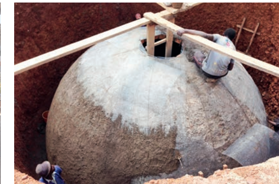
ECD&F Centres A 35000L underground rainwater tank provides water for the greater community's daily use
