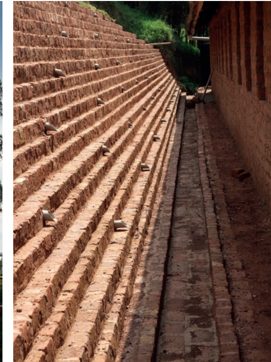
Lake Bunyonyi Secondary Various slope stabilisation measures have been put in place to mitigate erosion and potential landslides
