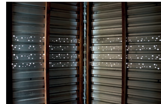
COF Primaries Polycarbonate is placed on top of perforated metal sheeting to allow light to enter while avoiding excessive glare
