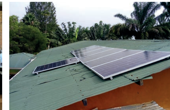
Standard solar photovoltaic cells mounted on a 15 degree pitched roof; an affordable, accessible and sustainable energy source
