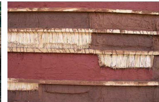
Living Tebogo by Base Habitat adapts vernacular wattle and daub construction (above) to produce a unique finish (below)
