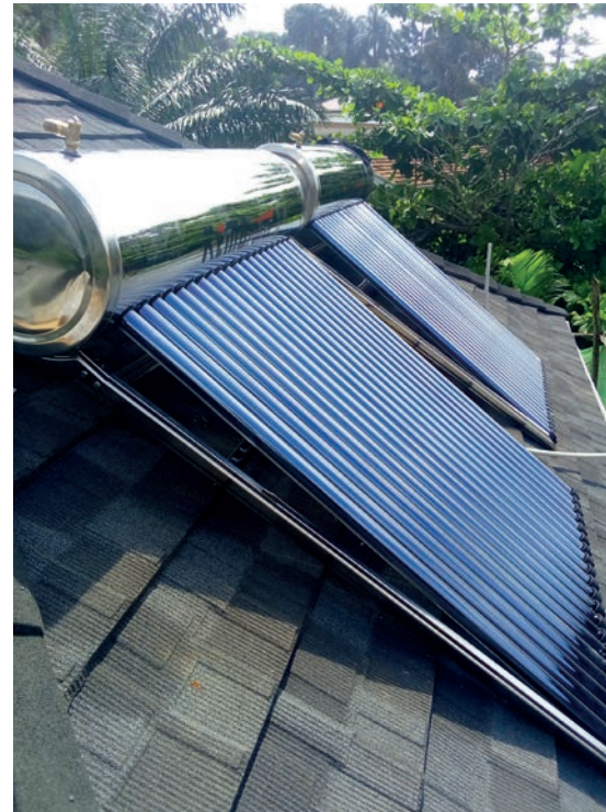
A professional solar thermal installation consisting of an evacuated tube solar water heater
