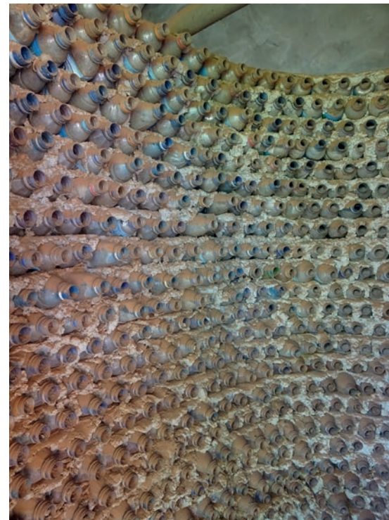
The Appropriate Technology Centre has constructed a toilet block out of recycled plastic bottles
